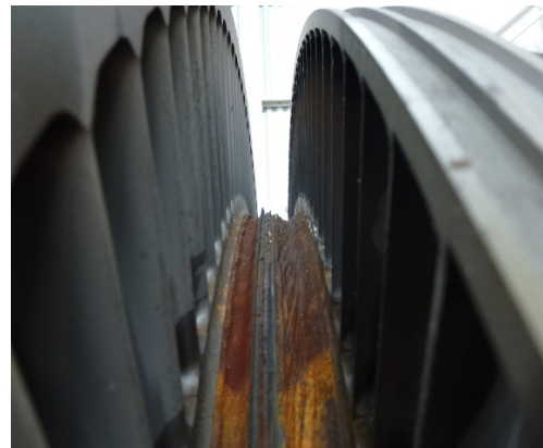
Figure 2 - Erosion at Interstage 3
