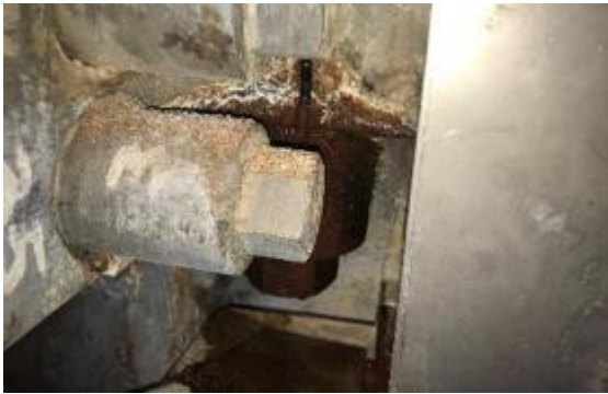
Figure 1 Casing half joint leak in operation
